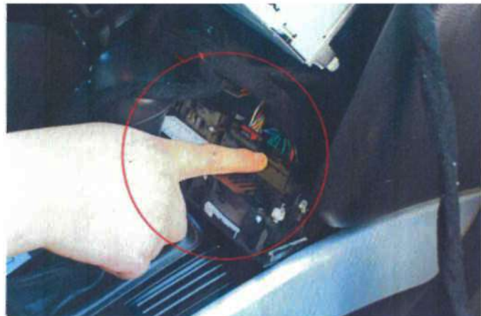
Transfer air conditioner panel plug
