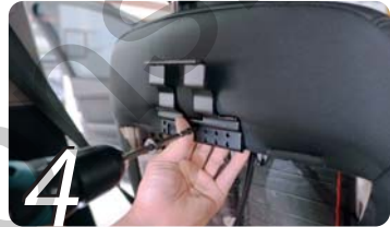
4 Fix the bracket on the seats frame by tightening the bolt(making a hole)
